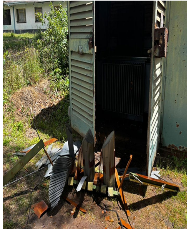
Some recent pictures of stolen conductor and vandalised substation.
