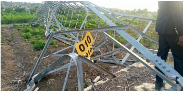
Recent picture of a vandalised transmission tower.
