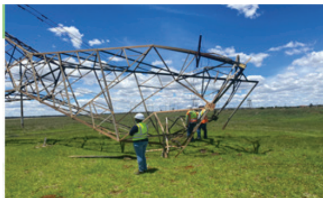
Figure 3: Vandalised tower in Eskom, South Africa
